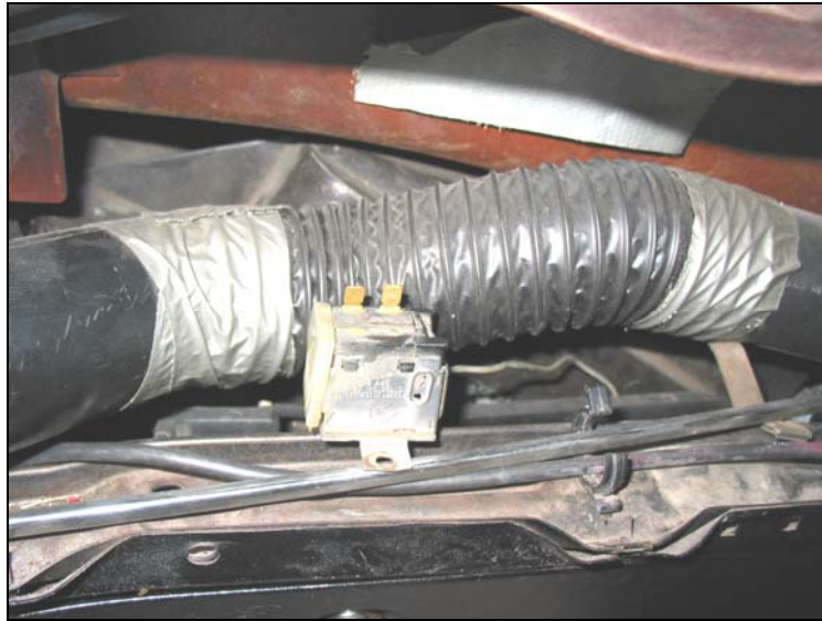
Figure 7-27 A/C De-Icing Switch
